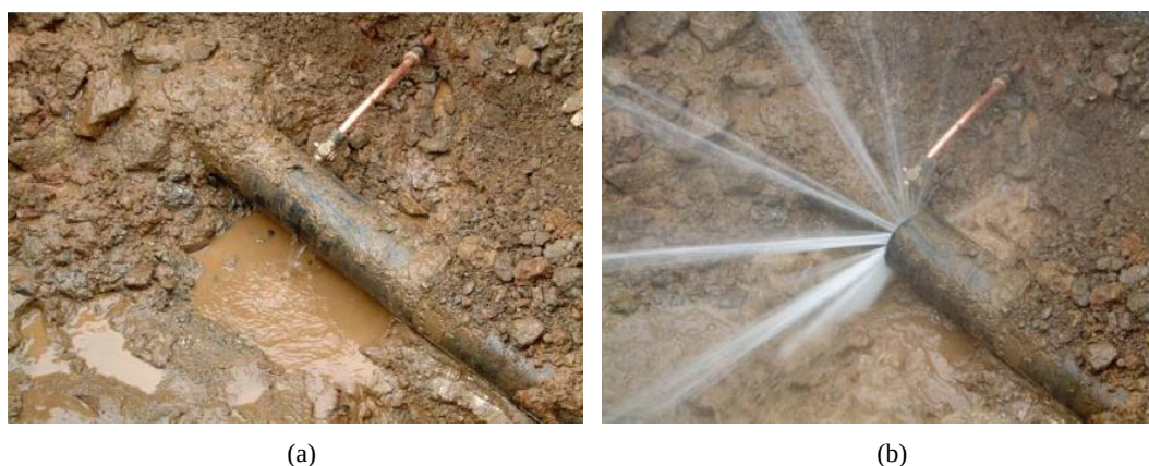
Figure 9. Leakage at various pressure situations (a) leak at low pressure and (b) leak at high pressure.
