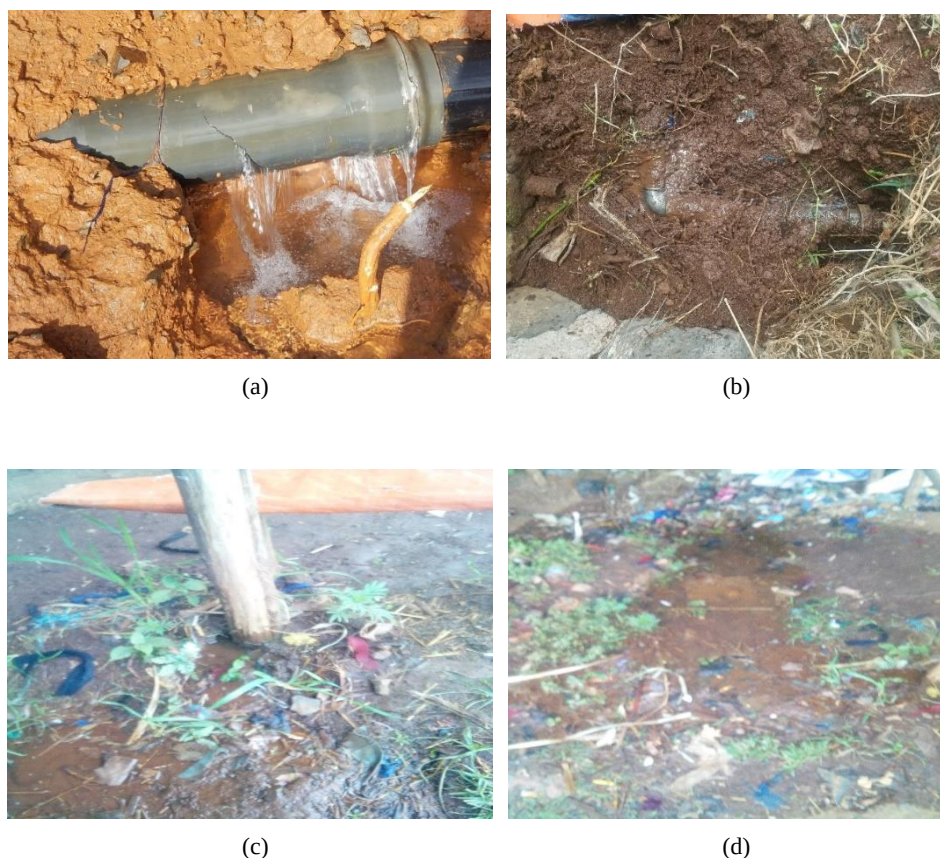
Figure 7. Leakage due to various factors: (a) damage of PVC pipe and followed by leakage due to collider development, (b) leakage due to detachment of aged iron pipe and rehabilitated iron elbow, (c) leakage due to poor HDPE fitting, and (d) flow of treated water over the earth surface.
