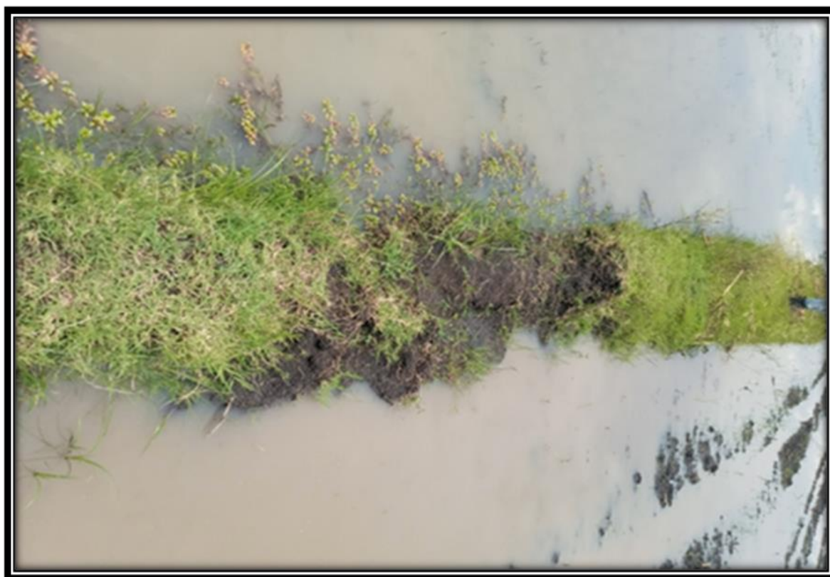
Figure 4. Broken Basin Bunds - The Bund Between the Two Basins is Thin and Collapsing.
