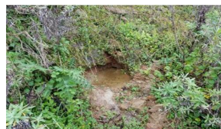
Figure 5. Groundwater/spring water indication at km 32+130.
