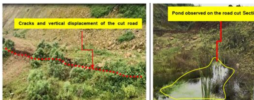
Figure 15. Cracks observed and water ponds in the given station.
