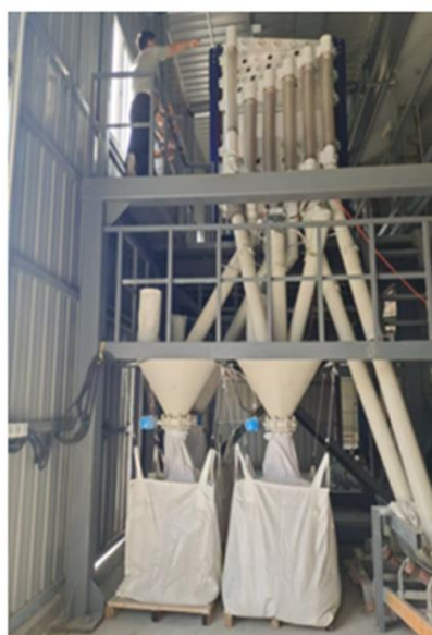
(b) Fine grading system
