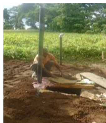
Figure 2. Vertical ventilation ducts.
