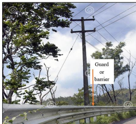
Figure 7. Typical guards near roadside MV line pole.
