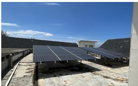
Figure 6. Solar Panel Placement.
