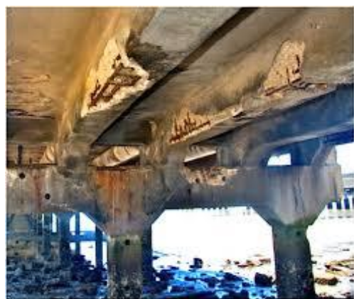
Figure 4. Damage because of wet.
