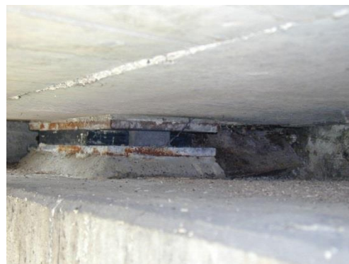
Figure 2. Pier metal rusting.
