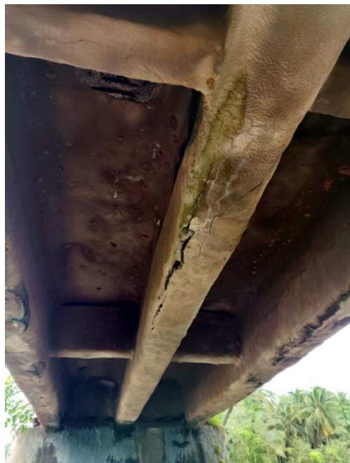
Figure 3. Bridge concrete part damage+ rushing.
