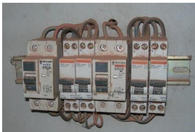
Figure 2. Dust deposition on circuit breakers [16].
