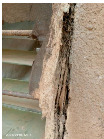
Figure 7. Termite damaged window frame in Ogbadigbo.
