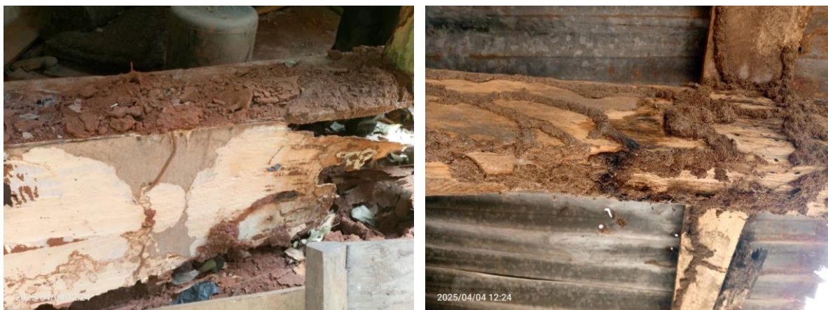
Figure 10. Roofing beam in a school severely infested with termites in Otukpo.
