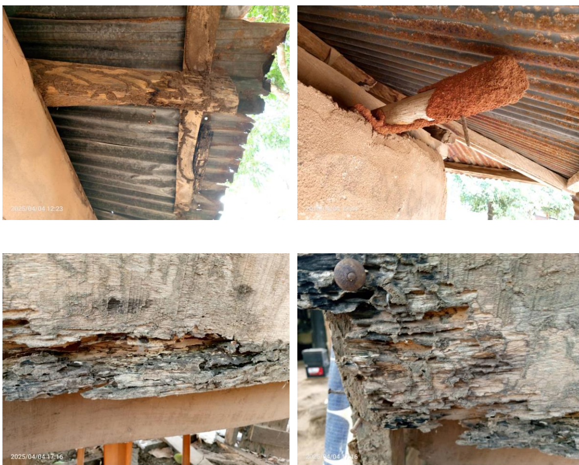
Figure 11. Roofing beam in a commercial building severely infested with termites in Makurdi.
