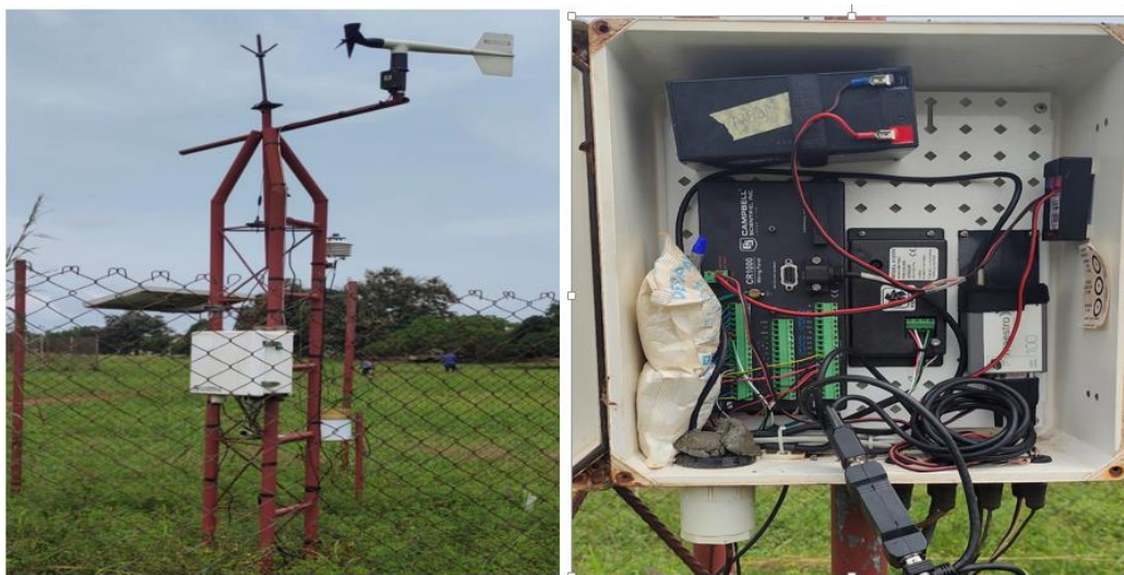
Figure 2. CAR_NASRDA Weather Station in Anyigba.
